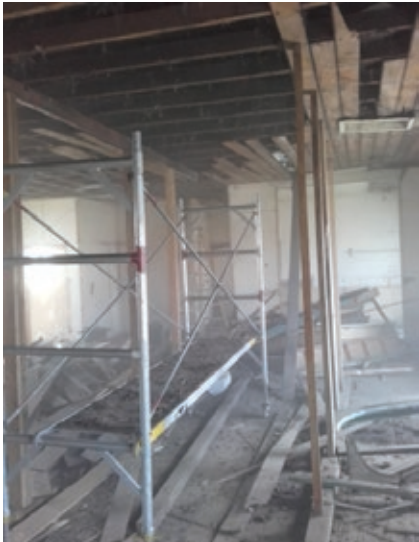
Inside the building, while the works were underway. Photo courtesy of Dave Hanan.
